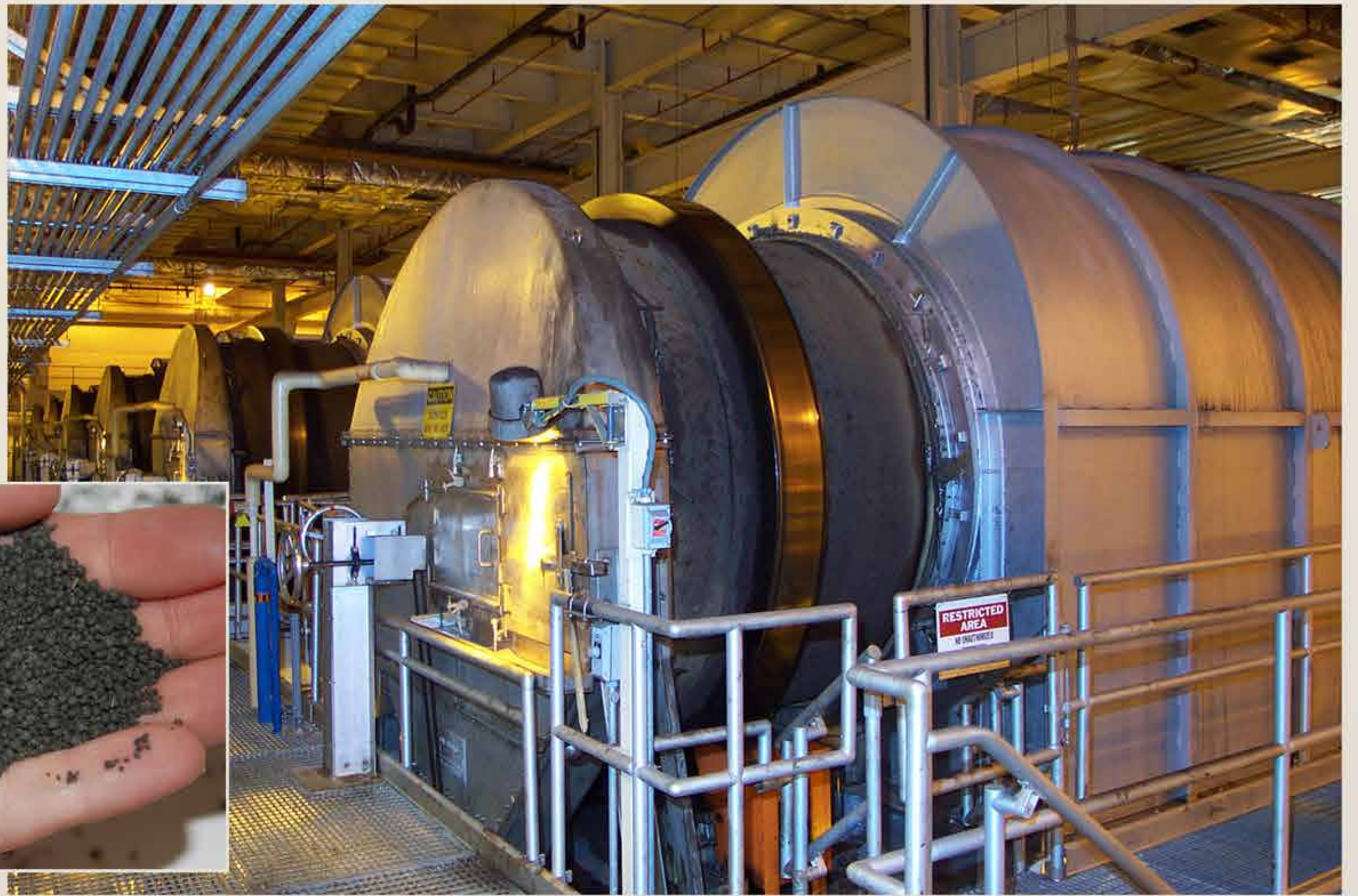
Milorganite Dryer Facility
